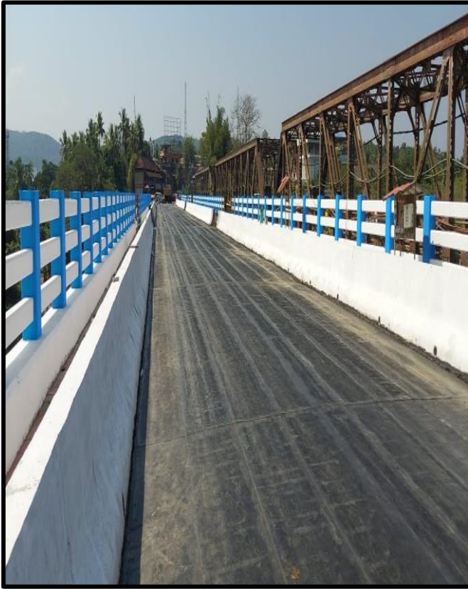
Water Proofing membrane fixing completed over the Deck slab of Iritty Bridge
