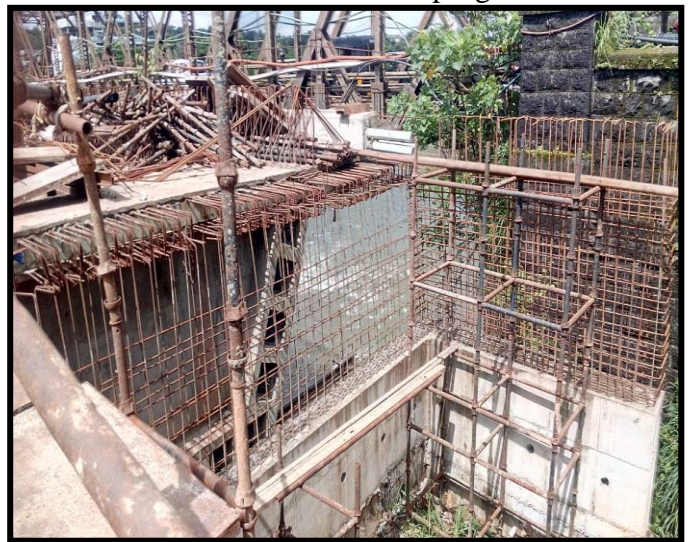
Iritty Bridge at km 42+198 Dirt wall A2 side reinforcement work in progress
