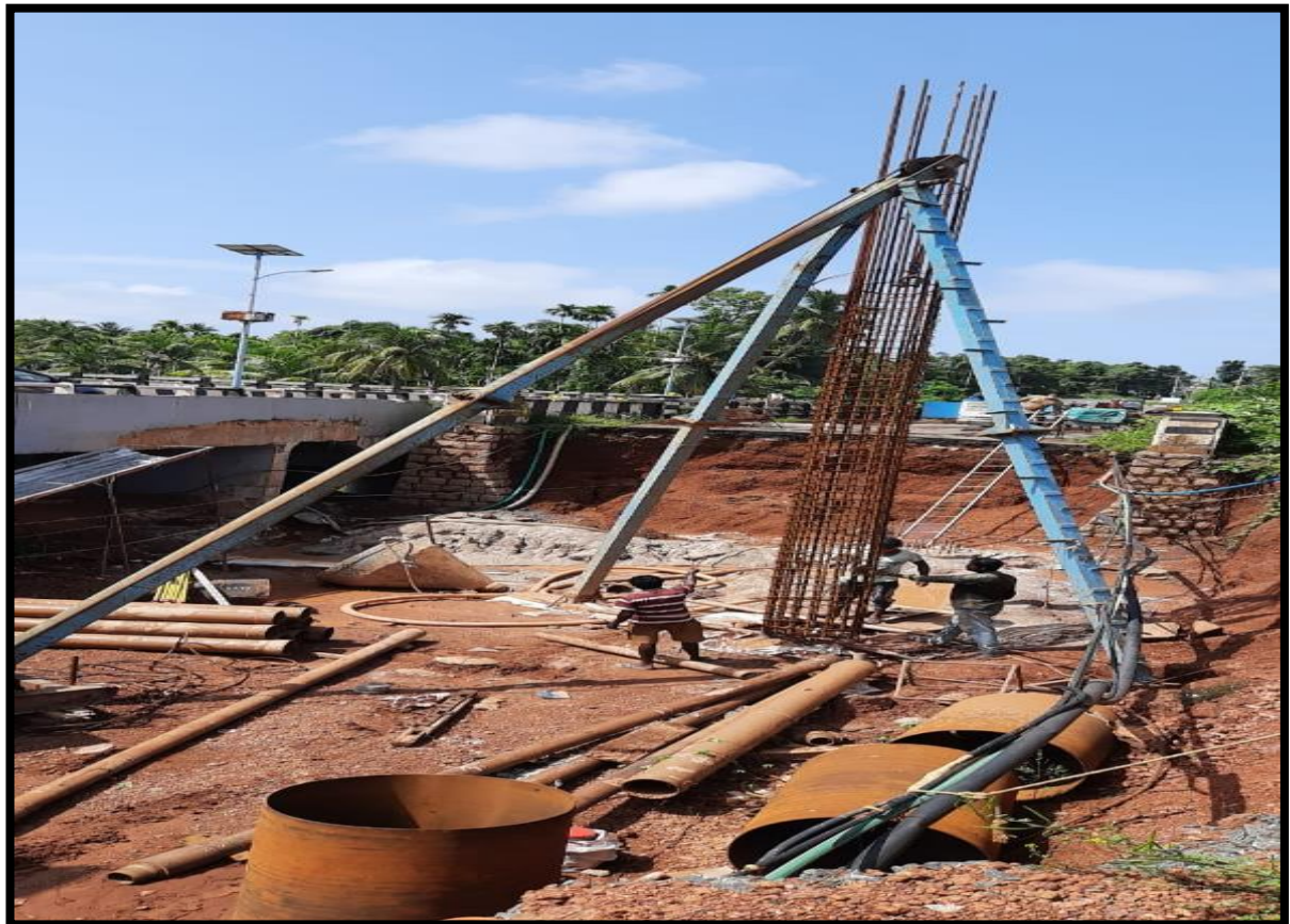
Ramapuram Existing bridge approach
