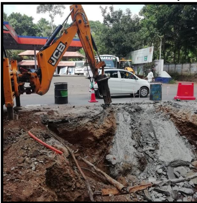
Dismantling of existing road cross structure work is in progress at Km 111+800.
