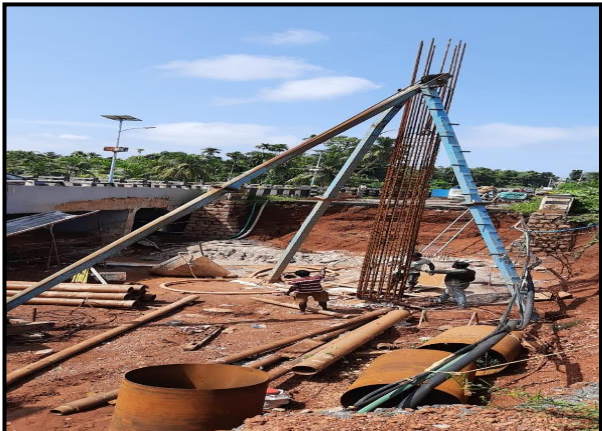
Ramapuram Existing bridge approach
